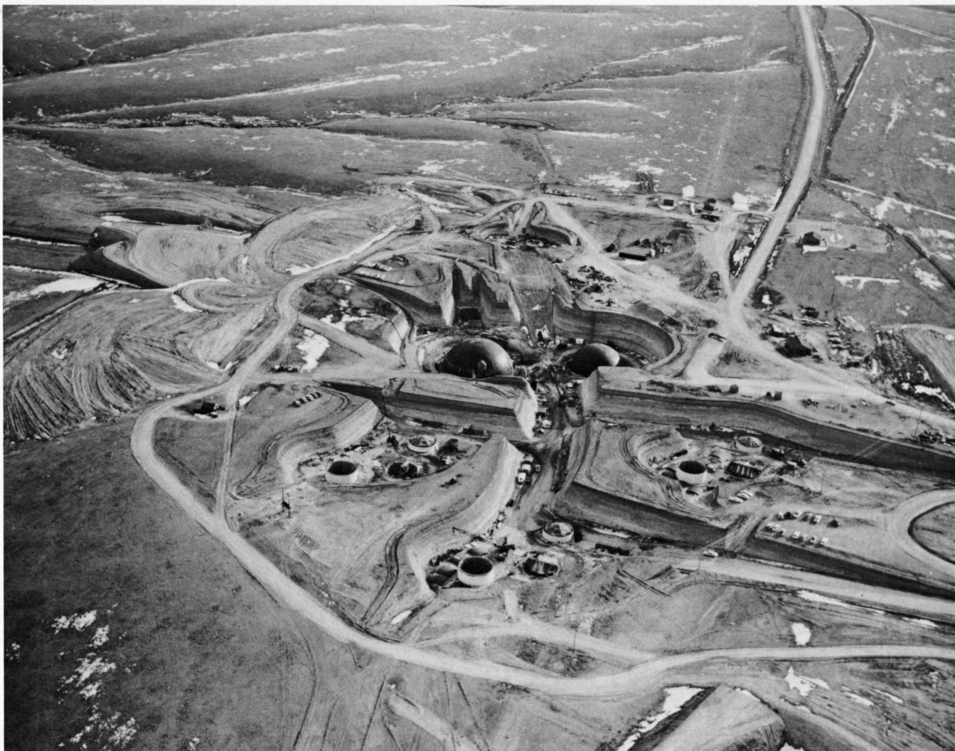
This view shows the domed powerhouse and control center for a Titan I missile complex under construction.
